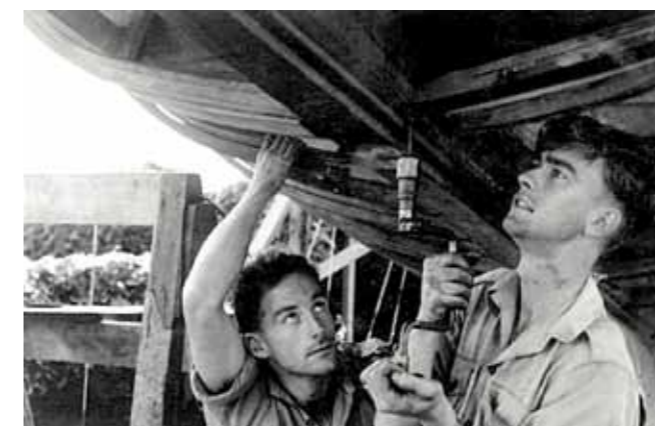
The author, aged 20, (at right) with Leda's co-owner, Sandy Wilson, working on the building. I was one of a rag-tag volunteer team, most of us reporters from the Auckland Star newspaper.
